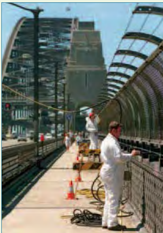
figure co.10 The Sydney Harbour Bridge is a 53 000-tonne steel structure protected from corrosion by paint. This is a continuous process that uses 90 000 litres of paint per coat.
